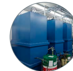
Tanks for bulk liquids that are pumped out to hose reels, and the transport of waste liquids.
