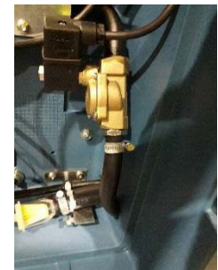
Compressed air connected
