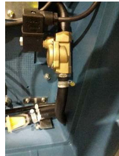
Hose connected to the valve
