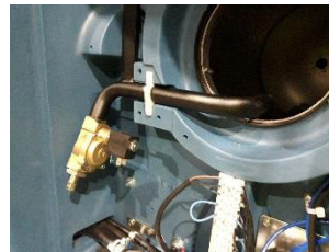
Compressed air supply pipe with the joint
