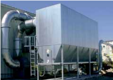
NFK Typical Ground Mounted
