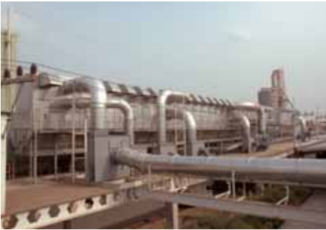
NFK located on roof, extracting from 2 factory
