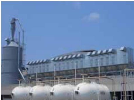
NFK blow into silo via transport fan
