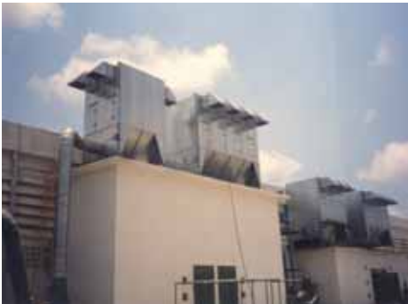
NFS dumping into building
