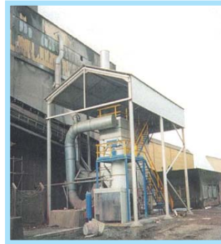
Conveying and handling hydrated lime for steel production
