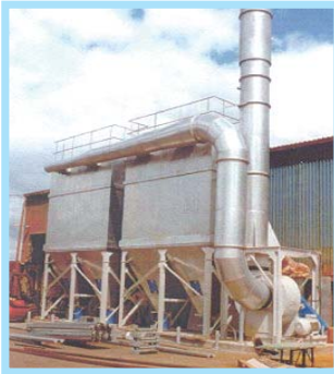
Fume extraction from hot-dip galvanizing process
