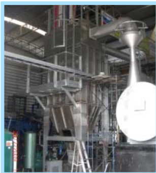
Waste gas cleaning for garbage disposal plant separating of dust and sulphur dioxide
