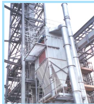
Dockside handling, conveying and storage, of grain
