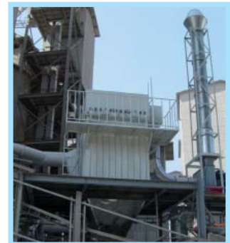
Cement Plant / Belt Conveyor Process, Cement / Lime industry
