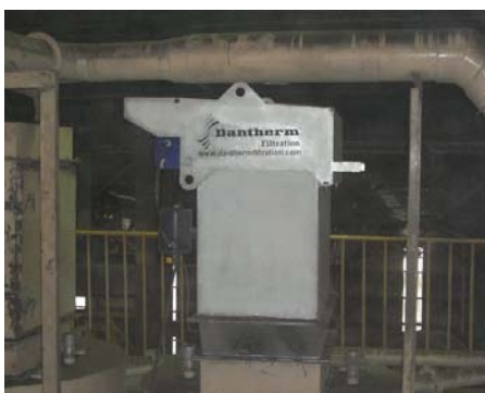
Silo venting system for additive silo, Foundry Industry
